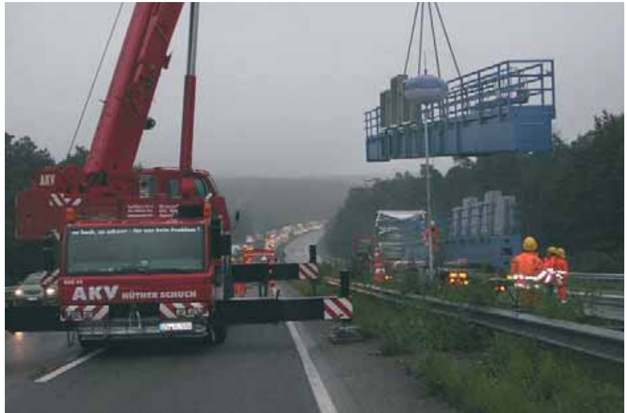
The gantries were fitted in just 15 minutes while the motorway was shut down either way.
